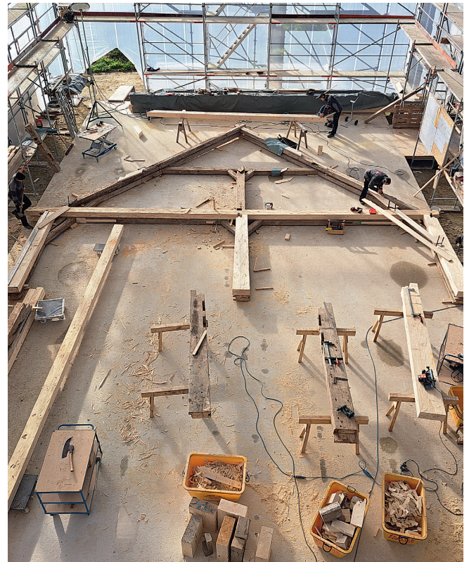
The barn is being dismantled into individual parts under a self-erected weather protection roof and stored carefully.
